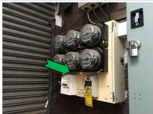
Photo 12. Interior, storage corridor, north end, east wall, electrical board – suspected non asbestos-containing bituminous material.
