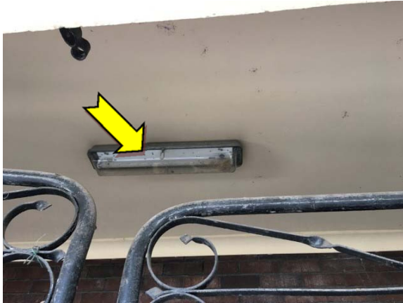
Photo 13. Exterior, east elevation, single tube fluorescent light fitting – suspected PCB-containing capacitor.
