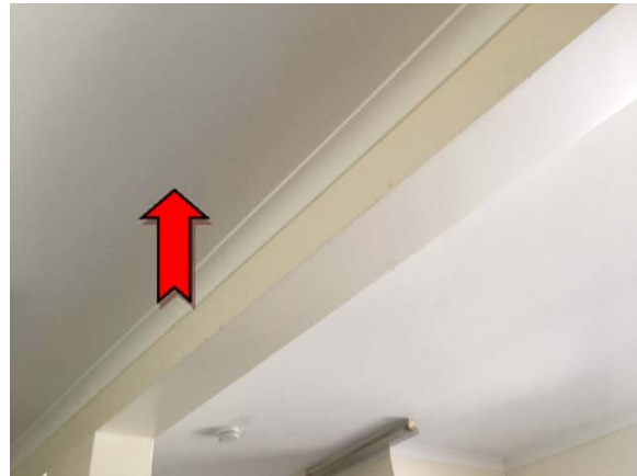
Photo 8. Interior, throughout, ceiling – suspected asbestos-containing fibre cement sheeting.
