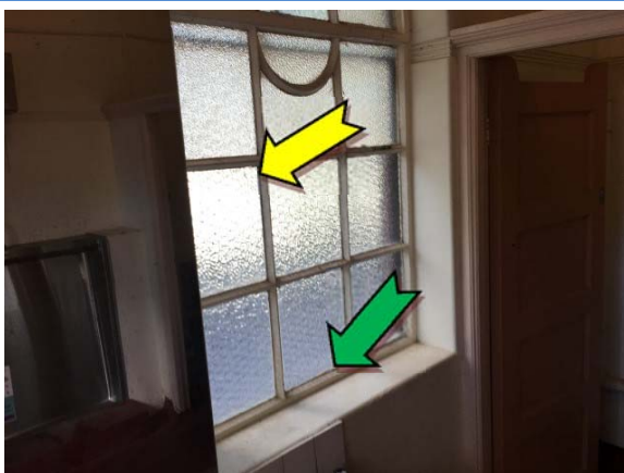
Photo 11. Interior, throughout, window frames – non asbestos-containing window caulking and suspected lead-containing beige upper paint systems.
