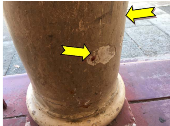
Photo 16. Exterior, columns – lead-containing white and yellow lower coloured paint systems and suspected lead-containing beige upper paint system.
