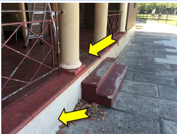
Photo 17. Exterior, throughout lower level walls and floor – suspected lead-containing red and white upper coloured paint systems.
