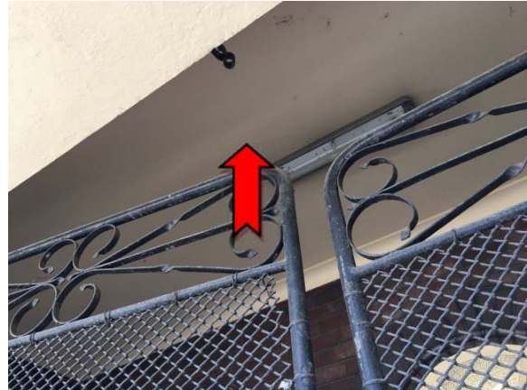
Photo 2. Exterior, east elevation, awning – suspected asbestos-containing fibre cement sheeting.
