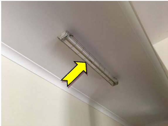
Photo 15. Interior, throughout, double tube fluorescent light fitting – suspected PCB-containing capacitor.
