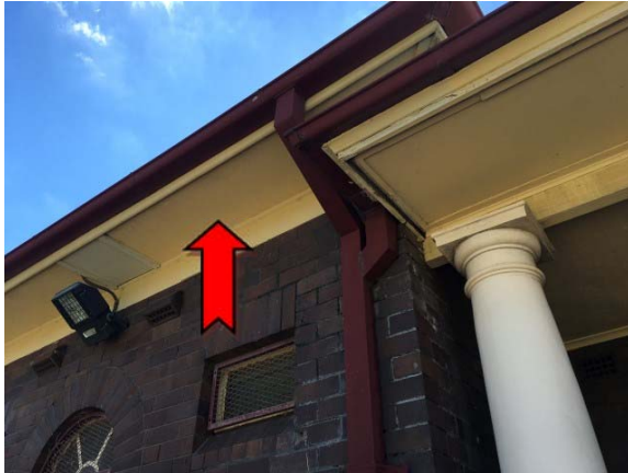
Photo 1. Exterior, eaves – suspected asbestos-containing fibre cement sheeting.
